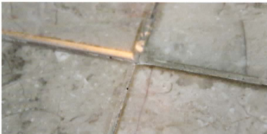
This warped tile was caused when this tile was manufactured.
